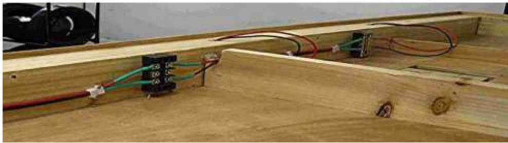
Open wiring and open connections occur when the unit is field assembled.
