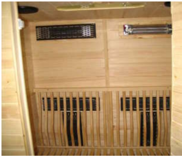
Metal cover plates are not bonded. Plate temperature exceeds the standard requirements.
